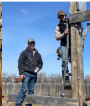
Trevor Ellingson (left) and Andy Arthur (right) install a barn camera system
