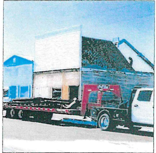
The original First State Bank building, one of the oldest structures on Timber Lake's Main Street, was demolished last week.
