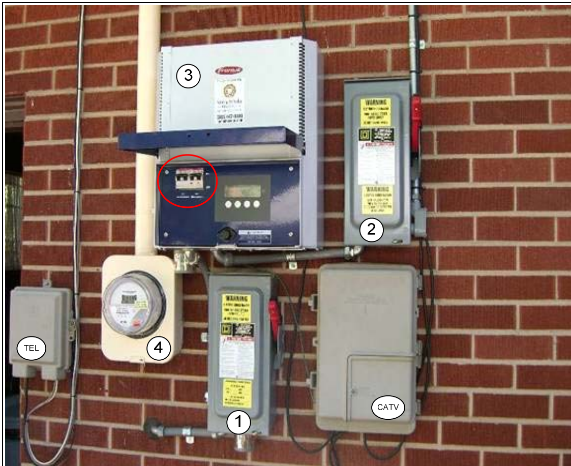
Figure 2. A typical residential PV installation includes (1) an EDS, (2) a DC disconnect, (3) an Inverter (with AC and DC breakers shown in the red circle), and (4) a revenue meter
