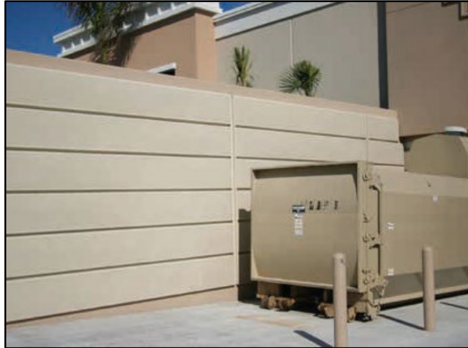
Figure 3a. Example of sound barrier (IAC Acoustics 2023).
