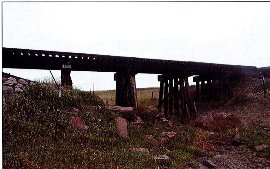
Figure 15. View of MH00002388 facing southeast. J. Larson 10/25/2016.
