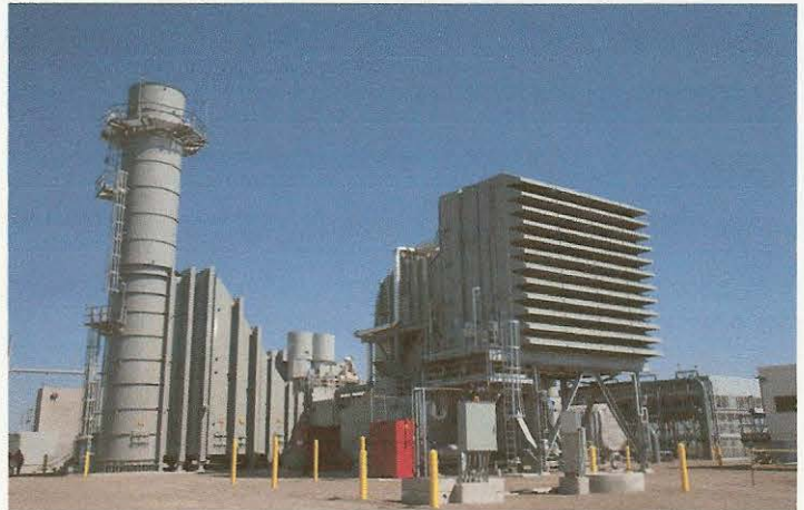
Culbertson Generation Station in Montana
