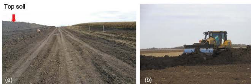
FIGURE 1 (a) Topsoil pile adjacent to the ROW zones. (b) The top soil was replaced by a Caterpillar D7E bulldozer after the exposed subsoil was tilled. The Caterpillar D7E fully loaded weight was 256 kN. Each track had a nominal track contact length of 3.02 m and a width of 0.76 m (Tekeste et al., 2019) [Colour figure can be viewed at wileyonlinelibrary.com ]
