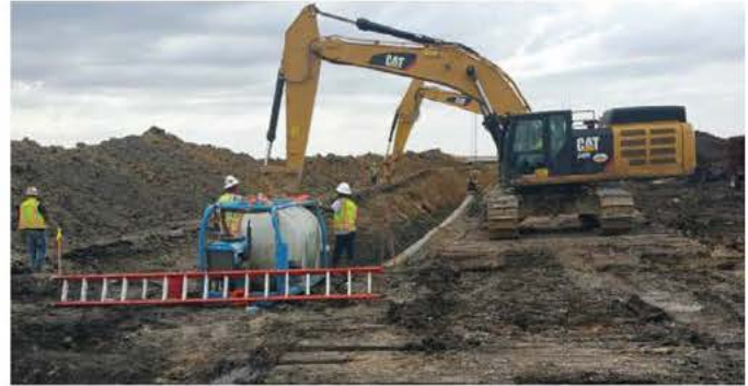
Caterpillar 349F hydraulic excavator. Fully loaded weight = 522 kN. Each track had a nominal track contact length of 5.36 m long and a width of a 0.76 m.
