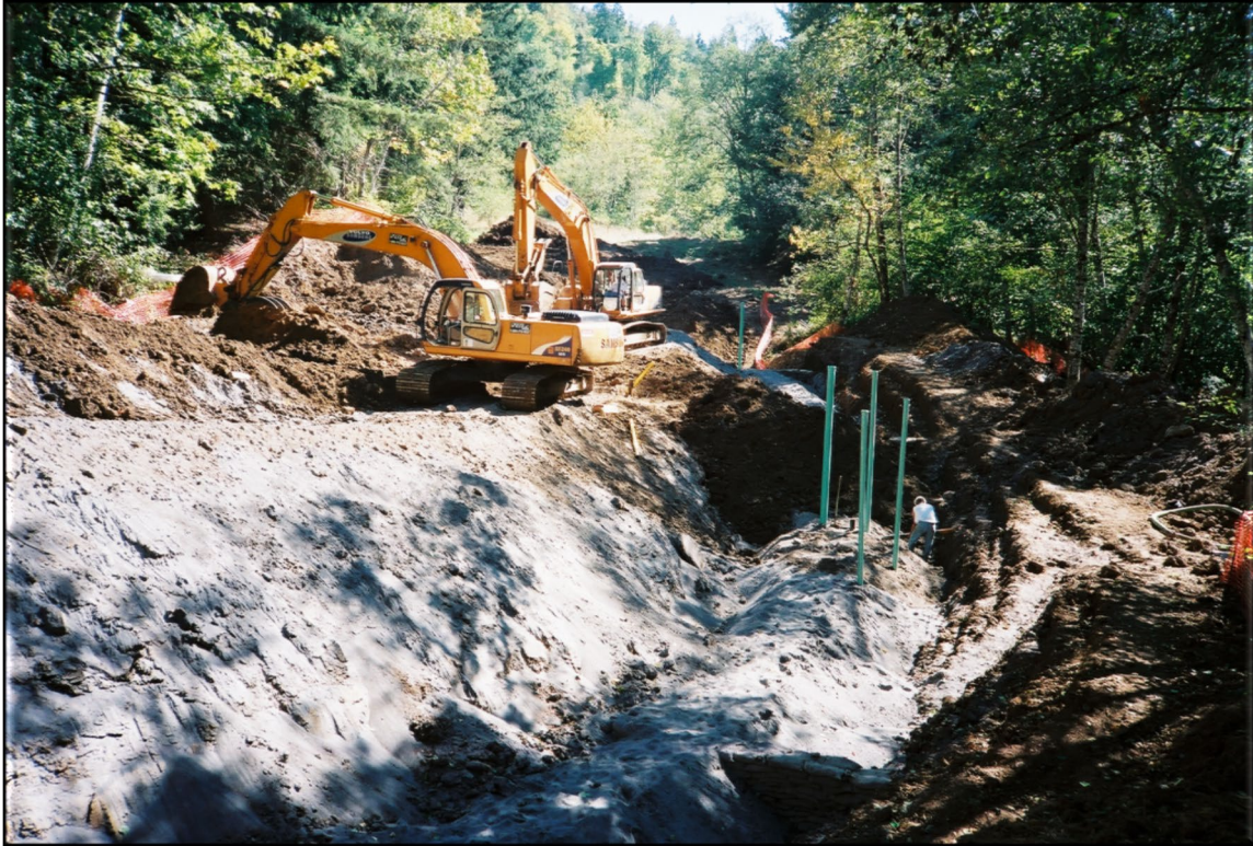
Figure 8-1. Select backfill (clean sand) being placed on and around a pipeline in a landslide in western Washington. The vertical piping was for inspection and cleanout (D. West, 2002 photo).
