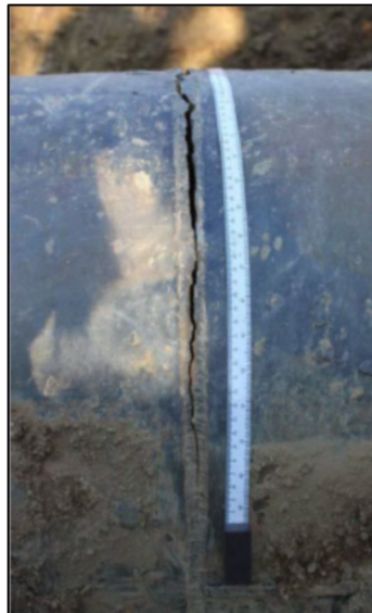
Figure 6-1. An example of girth weld failure
