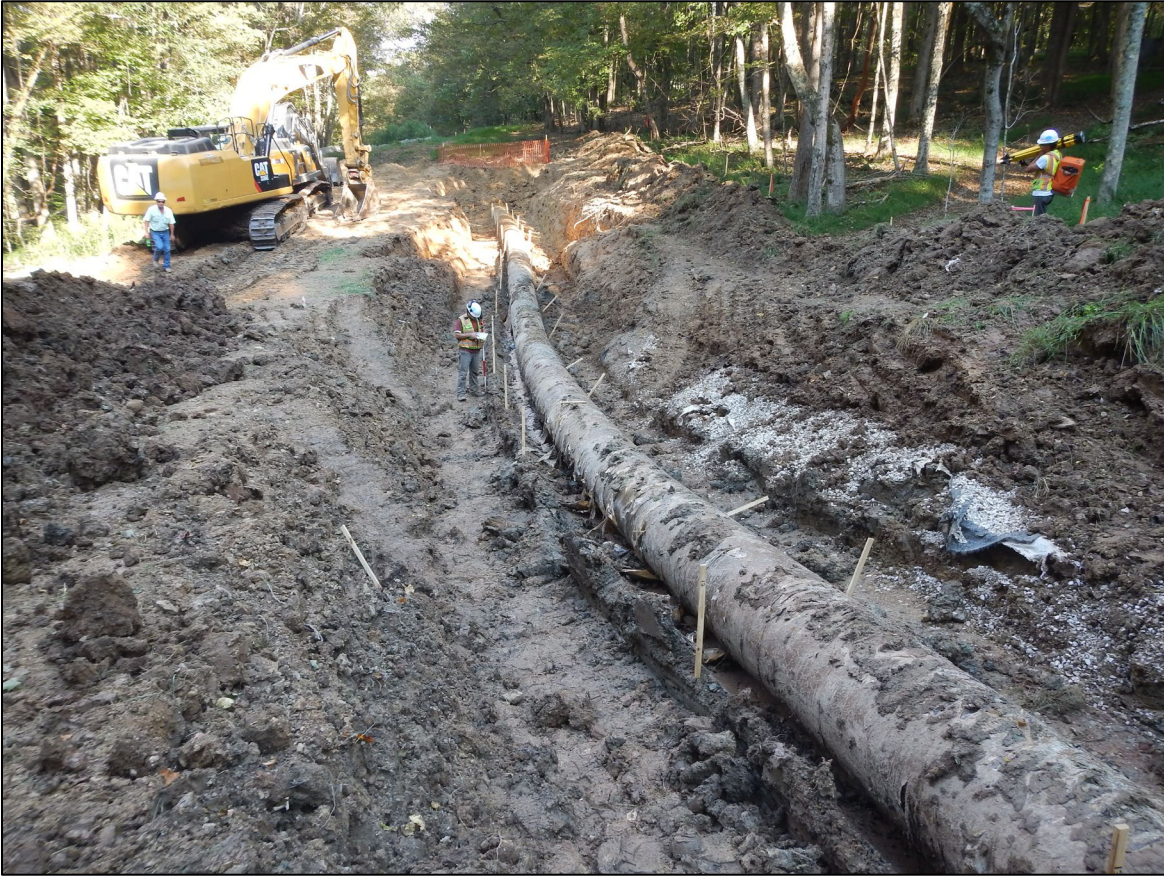
Figure 8-2. Stress-relief excavation of a natural gas pipeline showing pipe rebound and survey lathes placed to provide a visual reference to measure this rebound
