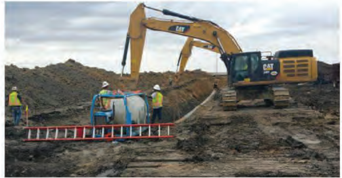
Caterpillar 349F hydraulic excavator. Fully loaded weight = 522 kN. Each track had a nominal track contact length of 5.36 m long and a width of 0.76 m.
