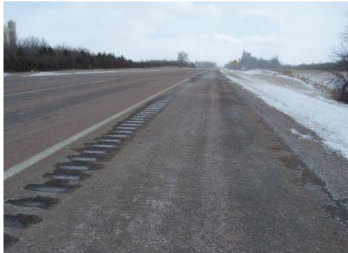
Eight foot wide shoulder with rumble strip (SD 11) - Accommodates all transportation and recreation modes on an other principal arterial, designated bicycle route
