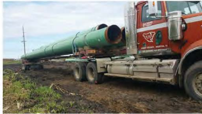
Semi-trailer truck with three pipes (each pipe was 24.4 m long, 0.76 m outer diameter, and 9.5 mm wall thickness).
