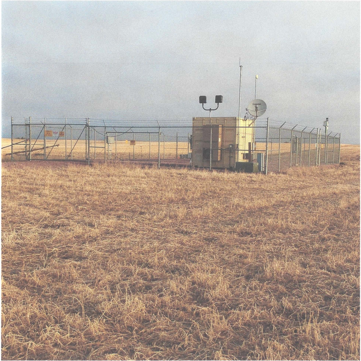
View of the Dakota Access Pipeline shut-off valve
