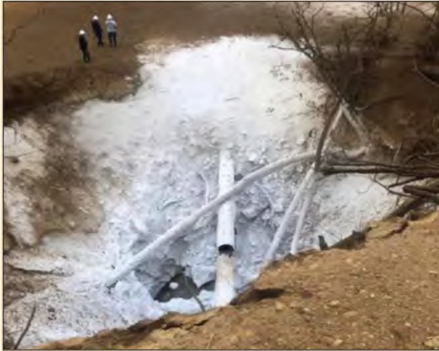
The Sartartia pipeline rupture. Source: Yazoo County Emergency Management Agency
