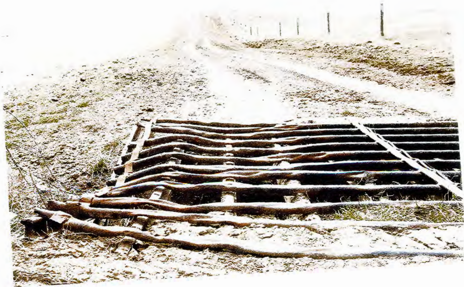
A cattleguard damaged during installation of the Bison high pressure gas pipeline in southeast Montana 04/12/2011
