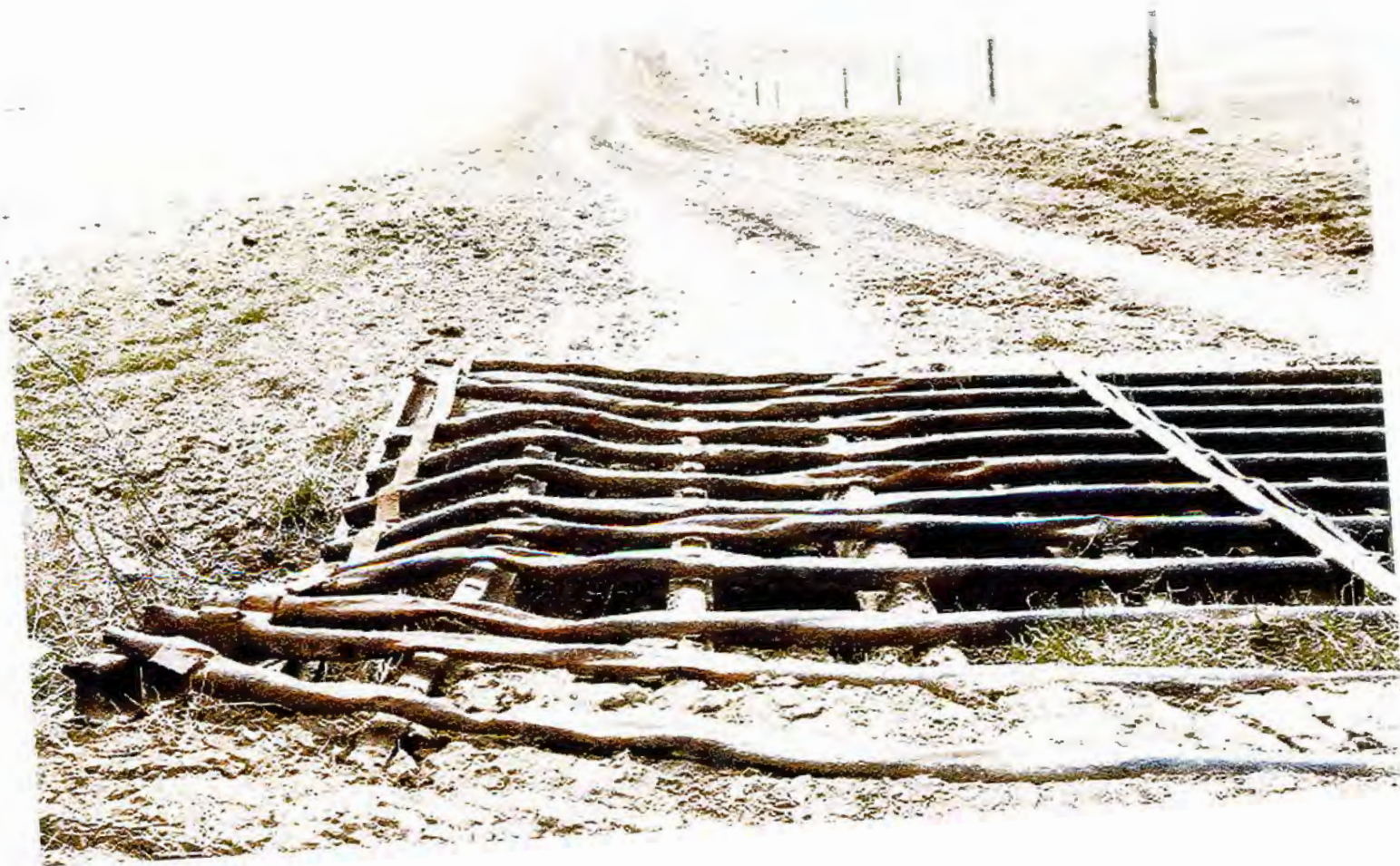
A cattleguard damaged during installation of the Bison high pressure gas pipeline in southeast Montana 04/12/2011
