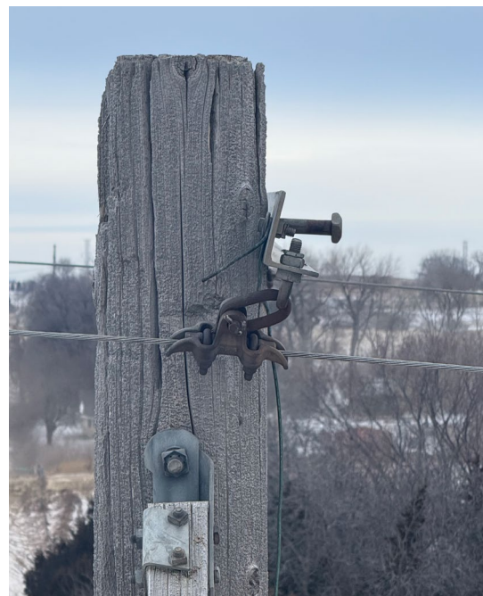
Example of loose hardware found during comprehensive structure inspection
