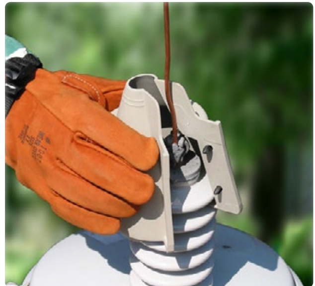
Figure 18: Example of wildlife guards on overhead equipment
