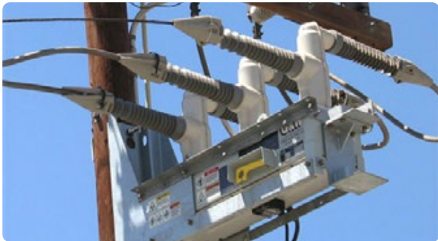
Figure 19: Example of distribution line recloser
