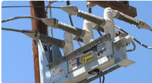
Figure 19: Example of distribution line recloser
