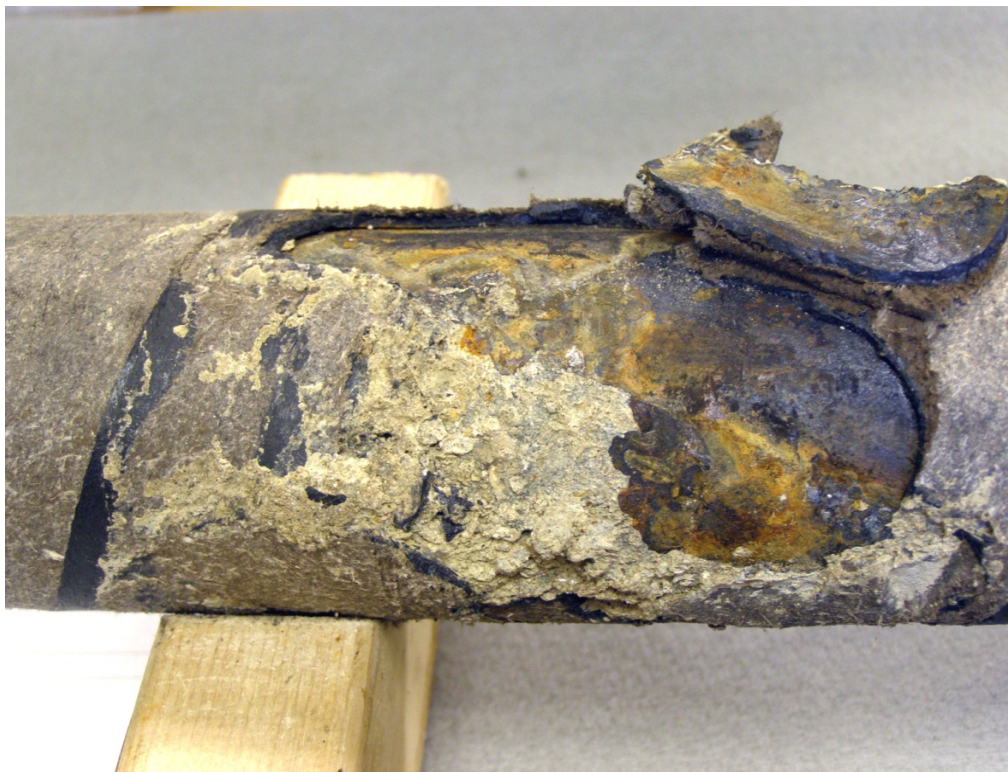
Figure 8. Disbonded area, side of pipe, located about 7 inches from End A
