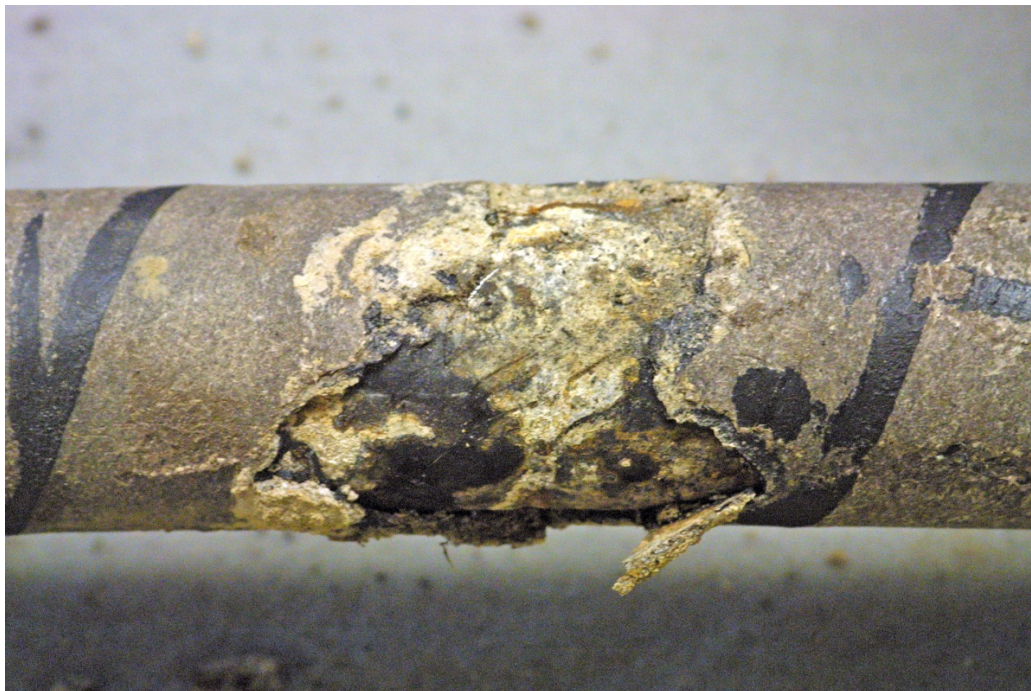
Figure 10. Disbonded area, side to bottom of pipe, located about 21 inches from End A
