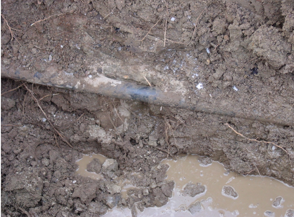
Figure 1. Pipe as initially exposed after the incident
