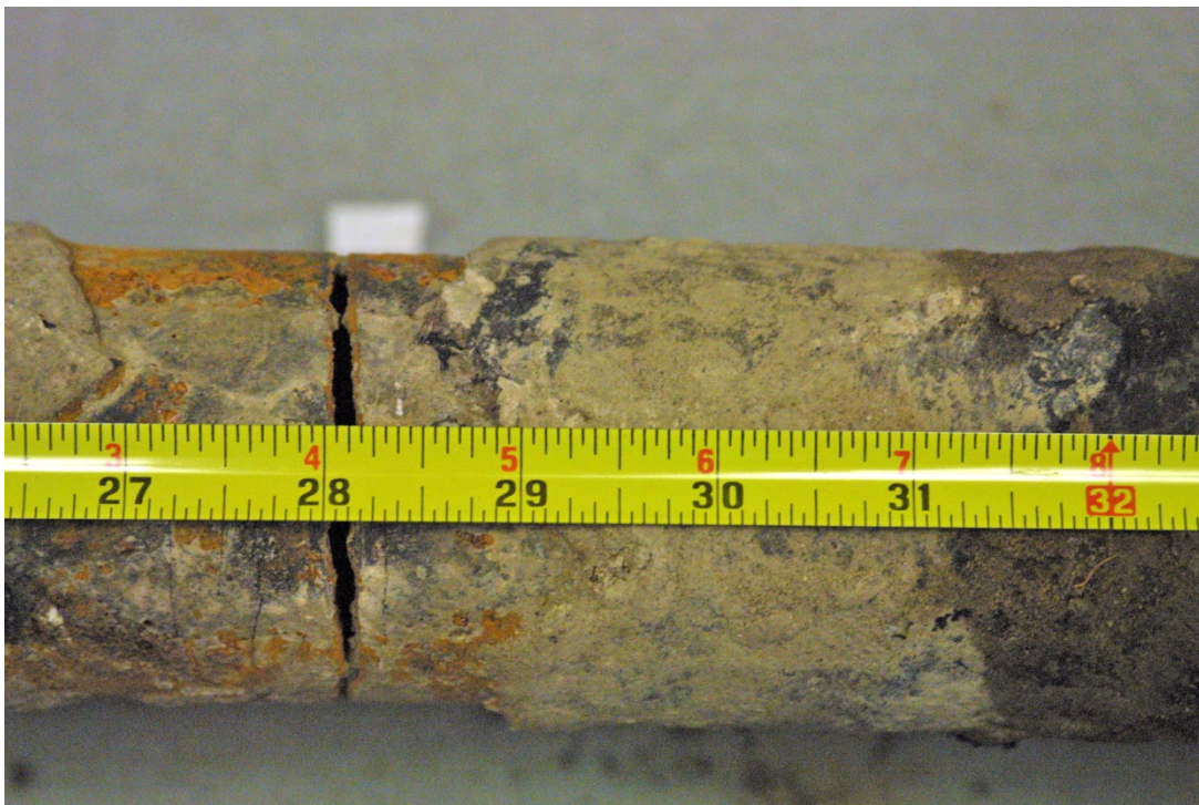
Figure 7. Circumferentially oriented crack located 28 inches from End A. The measuring tape in this photo is aligned with the bottom (6 o'clock position) of the pipe in service.
