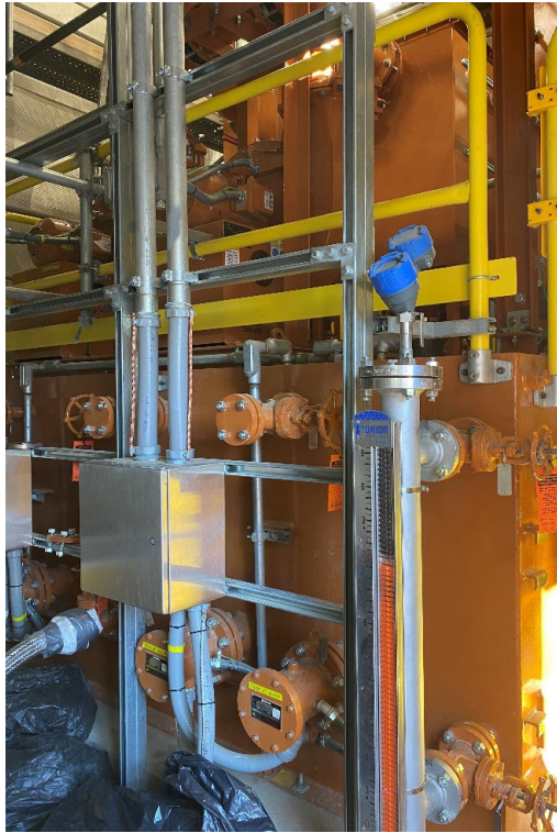
Lube oil reservoirs
