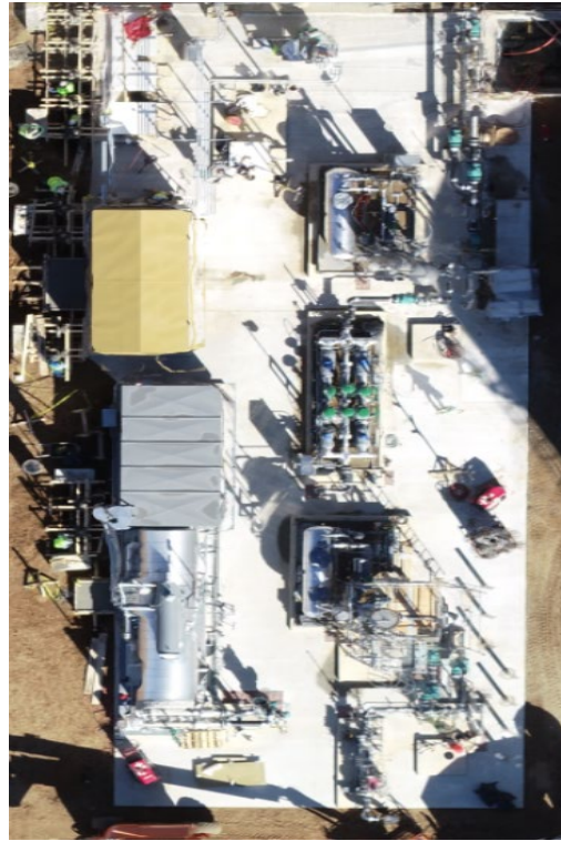
Gas Yard (natural gas leak)
