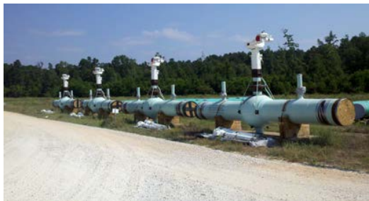
Figure 15: Valve Storage at Pipe Yard
