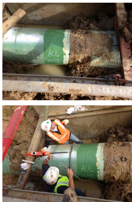
Figure 25 and 26: DCVG dig site (recoated)
