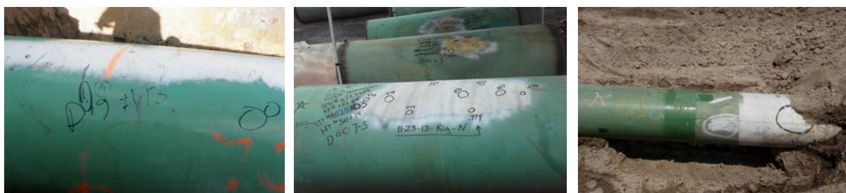
Figure 32, 33, 34 Examples of dents found with inspection tool.
