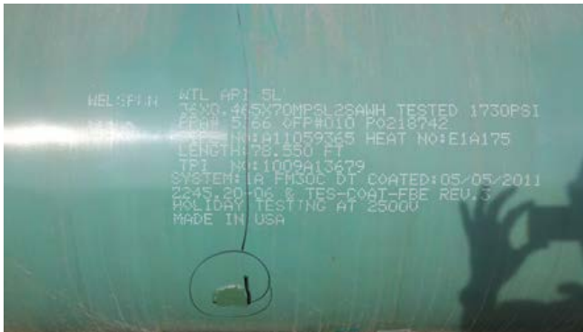
Figure 2: Pipe Specification Markings
